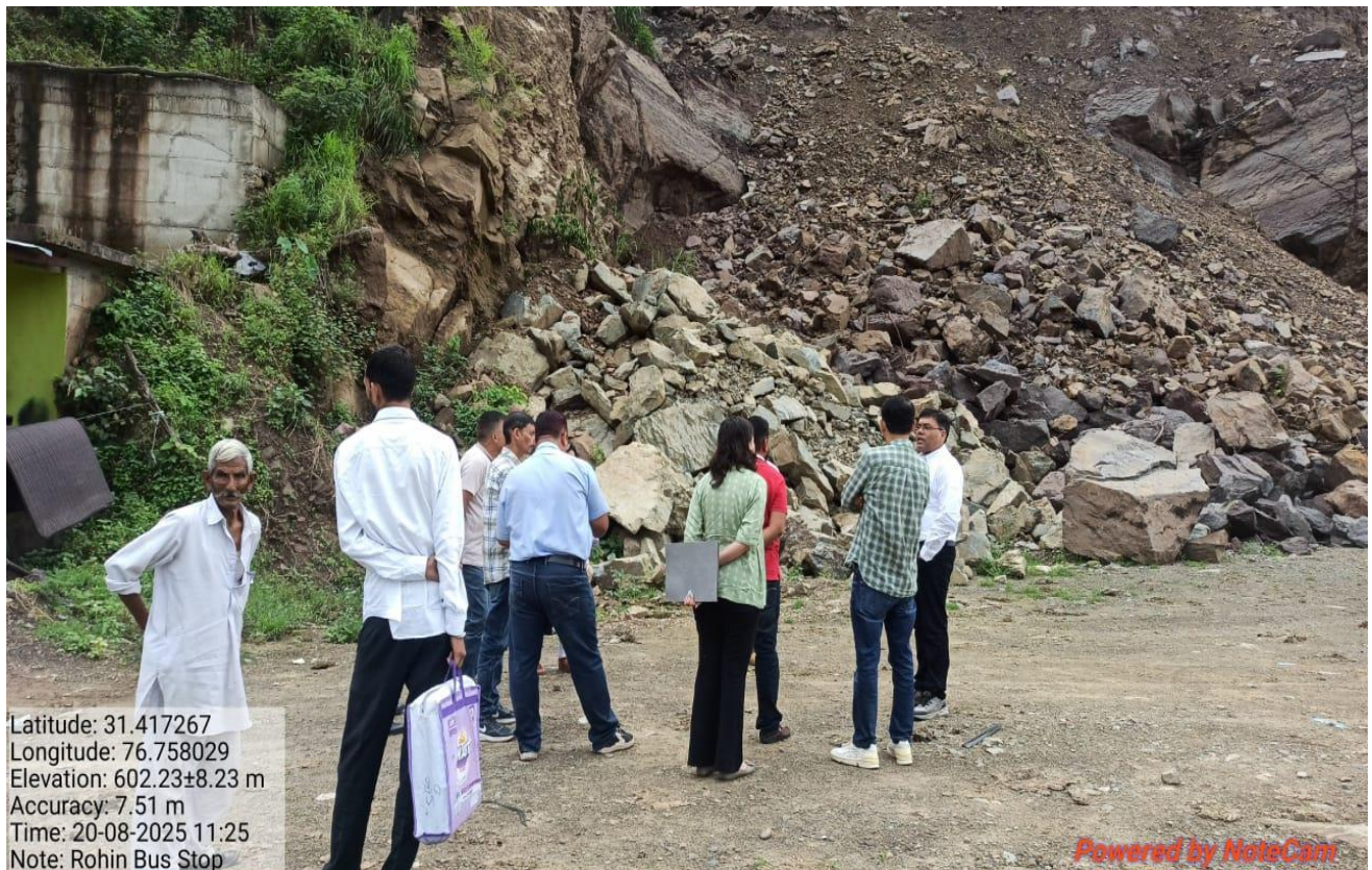
Photograph No. 02 : Direction Given By The Sub Divisional Magistrate To HPPWD Officials To Analyse The Quantum Of The Excavated Material.
